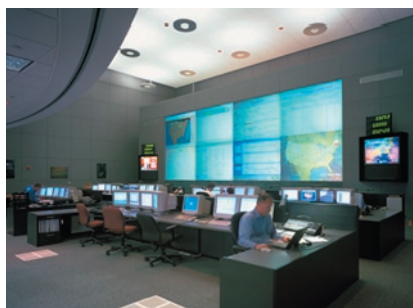
ERCOT Backup Control Center Austin, Texas
