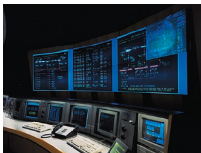
Xcel Energy Company World Class Control Room Minneapolis, Minnesota
